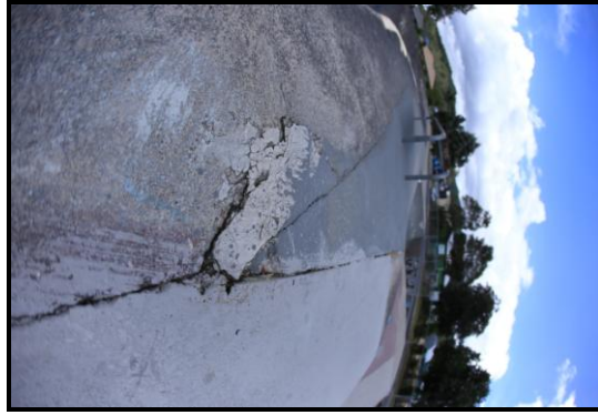
Figure 5. Old Repair Failing, Broken/Chipped Concrete.
