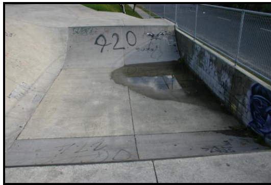
Figure 6. Water Pooling, From Poor/Blocked Drainage.
