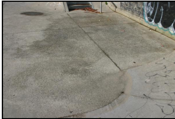
Figure 8. Rough Exposed Concrete
