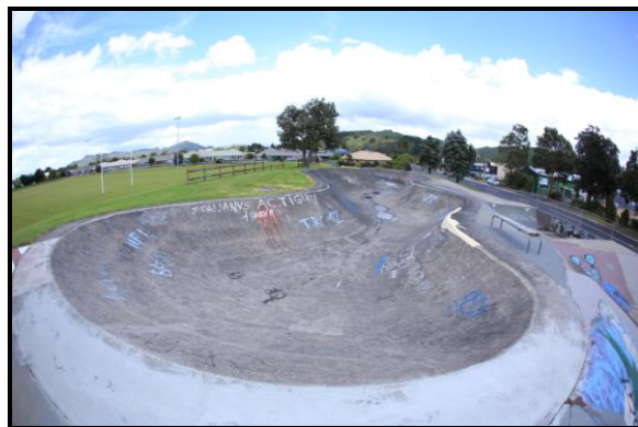
Figure 9. Rough Exposed Concrete
