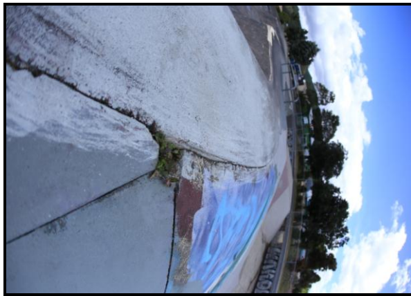
Figure 4. Damaged Concrete, Chipped and Broken Concrete Slab.
