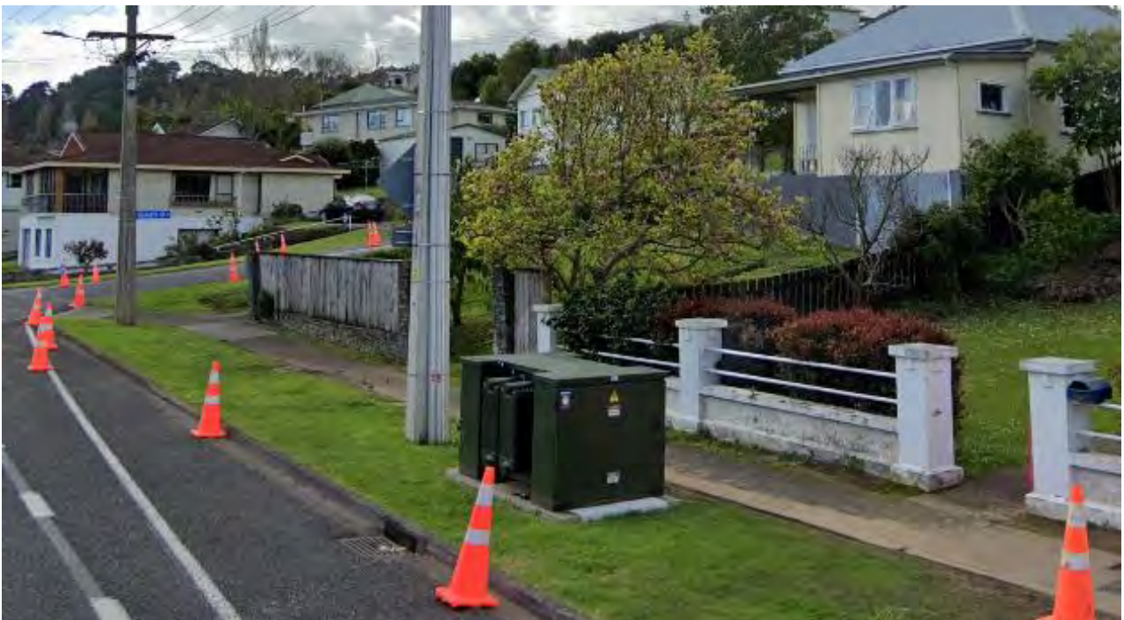
Figure 3-4: PowerCo Transformer on Rolleston Street
